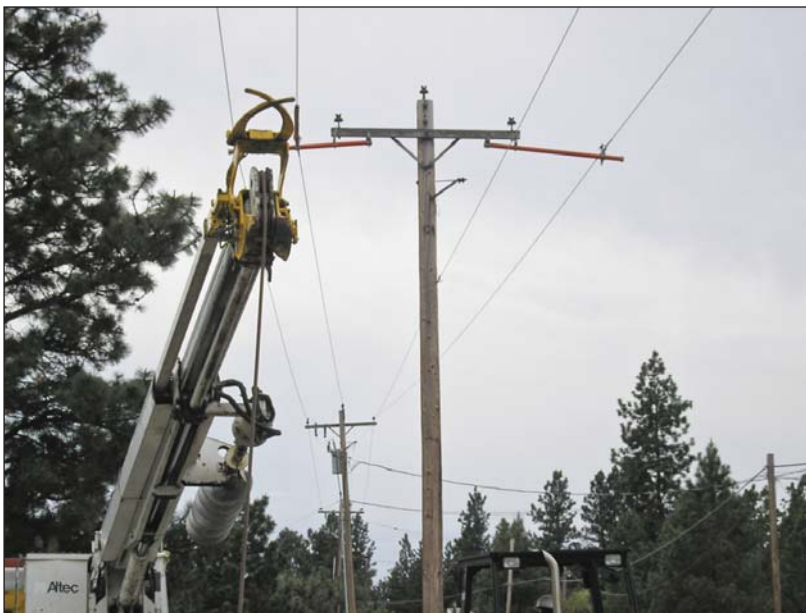
The energized conductors are on hot arms to give room to set the new pole.
