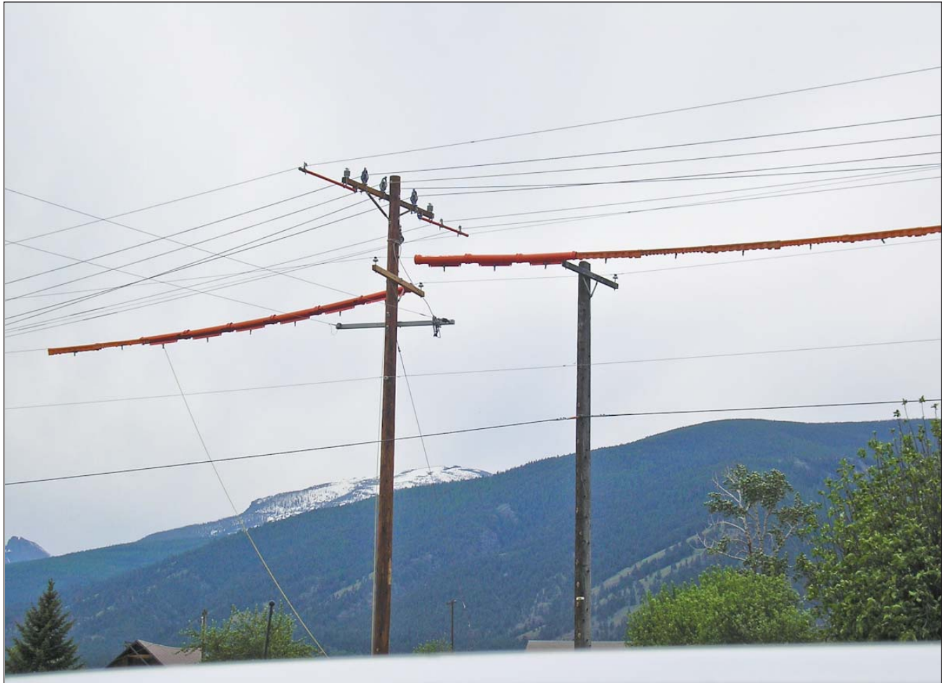
The energized wires are spread out and the new wires are inside the sheaves. The other line is energized and covered. This allows the Member's power to remain on while building the new line.
