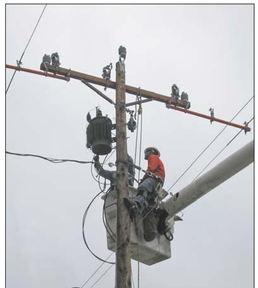
The new pole has been set and the Member's service is being reconnected.
